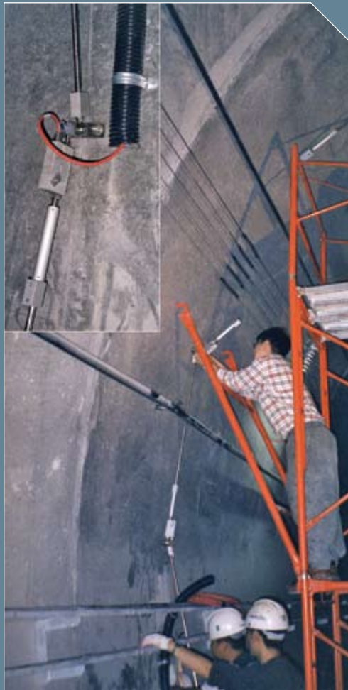
Typical installation of the RST Tunnel Profile System, with the inset photo showing a close-up of the final setup.
