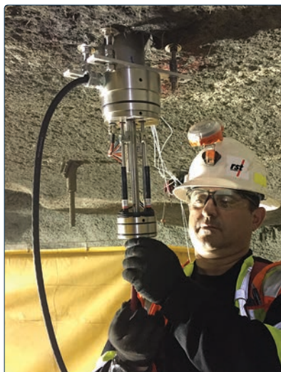
A Borehole Extensometer, with the Electrical Head cover removed, is being installed into the ceiling of an underground opening.
